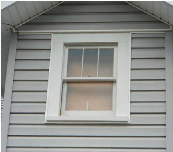
Siding Covers Dormer and Window Frame - Loss of Dimension, Profile and Decorative Detail
