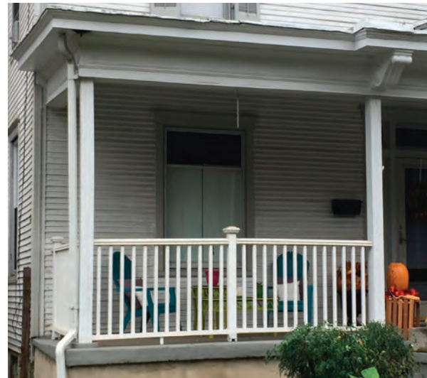
Replacement "Home Store" Porch Railing with Tall Height, Thin Balusters, and Synthetic Material
